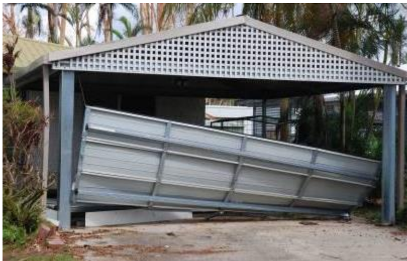
PICTURE 3-2 – OPENINGS DAMAGE
