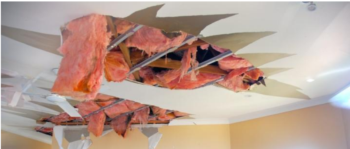
Figure 11. Wind driven rain damage to a modern (2000s) masonry block home as presented to builders, assessors, and engineers for experience based estimates of repair cost
