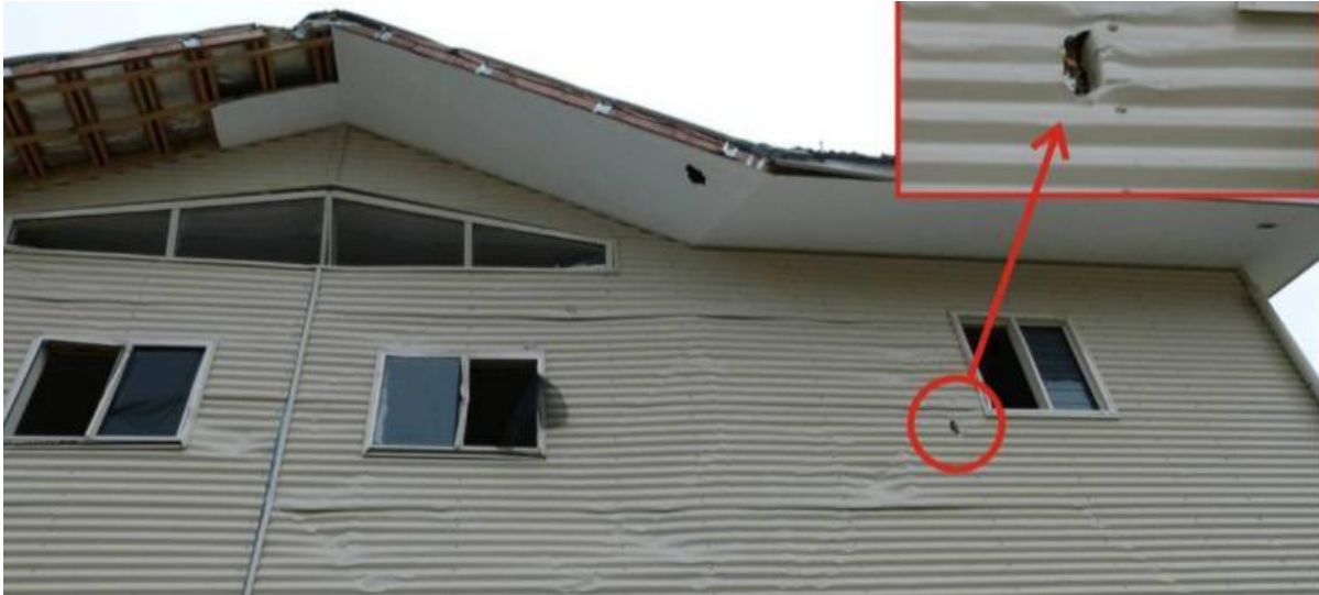
Figure 14. Wind driven debris damage to a modern home as presented to builders, assessors, and engineers for experience based estimates of repair cost
