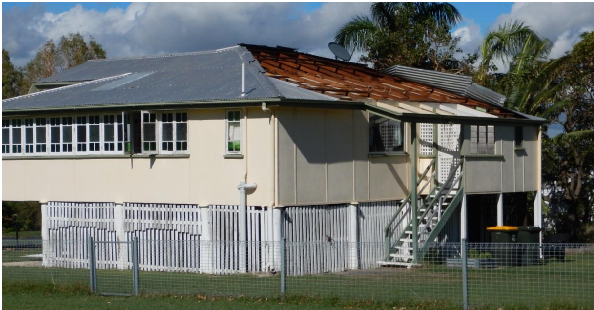
Figure 10. Wind-induced roofing damage to high-set 1920s home as presented to builders, assessors, and engineers for experience based estimates of repair cost
