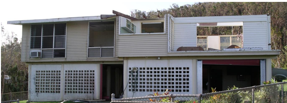
Figure 16. Roofing and wall damage to a high-set 1970s home as presented to builders, assessors, and engineers for experience based estimates of repair cost
