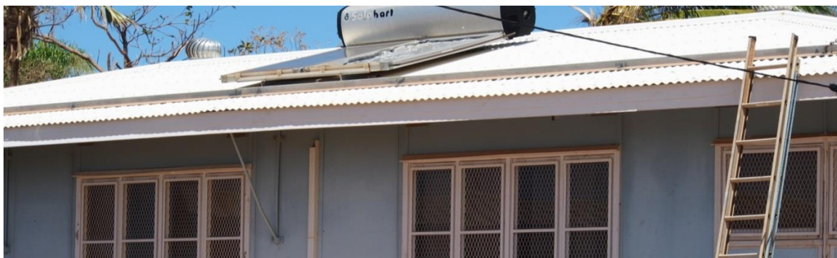
Figure 20. Drawing from Australian Standard's Handbook HB132.2 and Typical over-batten installation per HB132.2 Structural Upgrading of Older Houses
