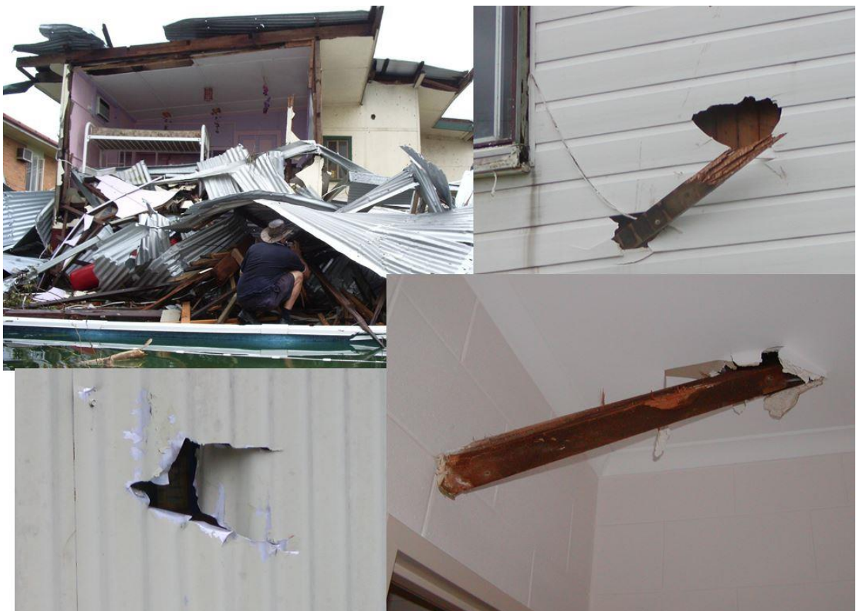
Figure 17. Wind-driven debris damage from structural failure of neighboring housing
