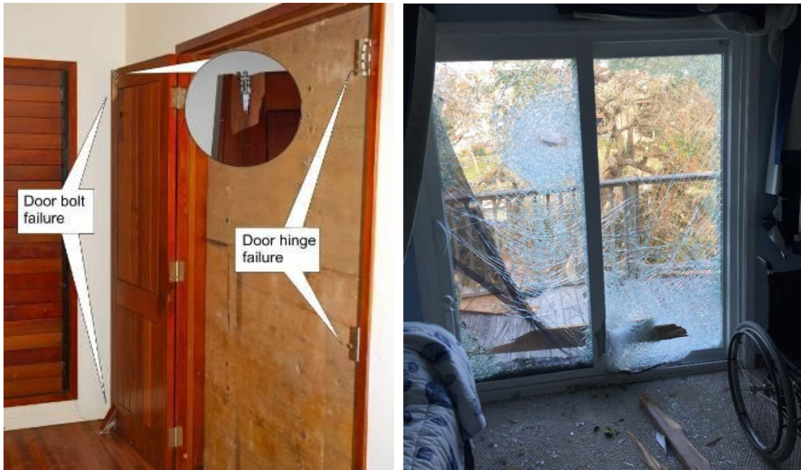
Figure 7. Door bolt and hinge failure from Cyclone Yasi in 2011 (left) and wind-borne debris failure of impact-resistant glass door from a tornado during Hurricane Harvey in 2017 (right)
