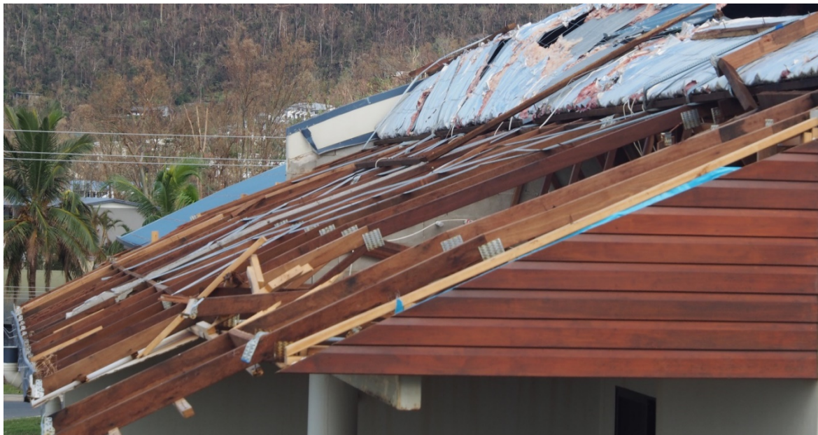
Figure 1. Severe roofing damage from Cyclone Debbie in 2017 due to inadequate load capacity at the batten to rafter connection
